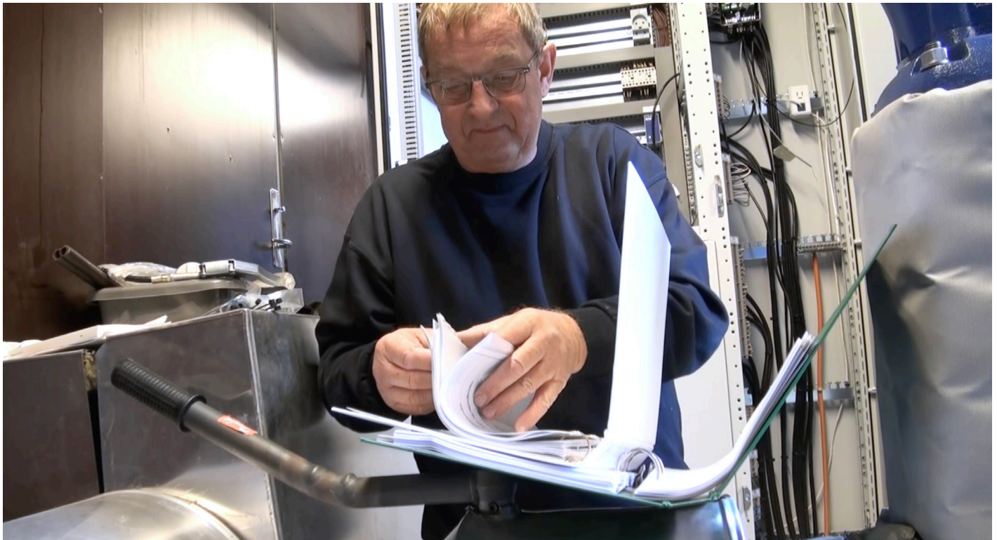
Jens Ole Olsen, foreman of Hirtshals Fjernvarme, installs an electronic surveillance monitor on a CR-95 pump at the Tornby pumping station.
